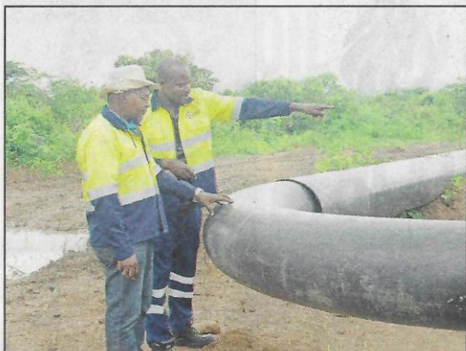
EACOP staff looking at the Kingfisher feeder pipeline near Ground Zero of the EACOP pipeline in Kabalega Industrial Park
